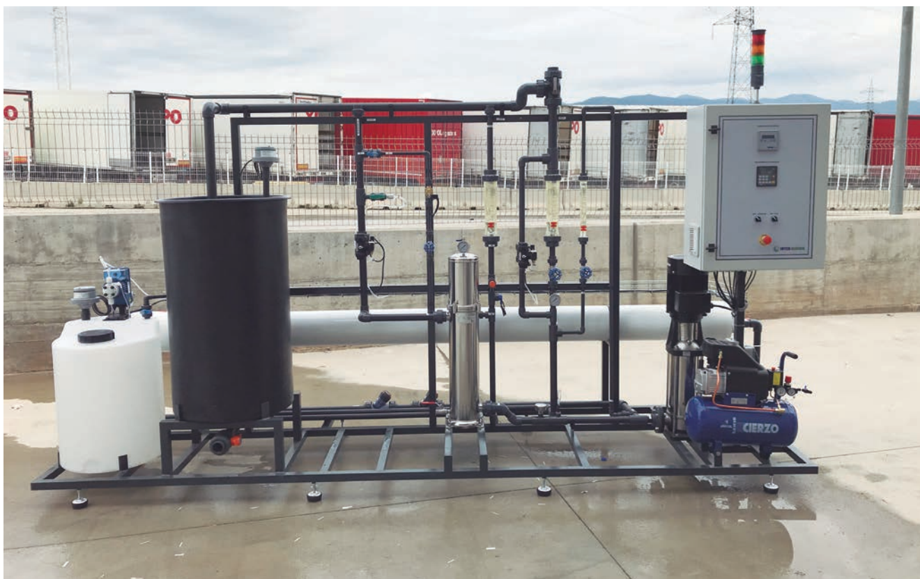
Industrial Reverse Osmosis of 60.000 l/day installed in Argelia.
