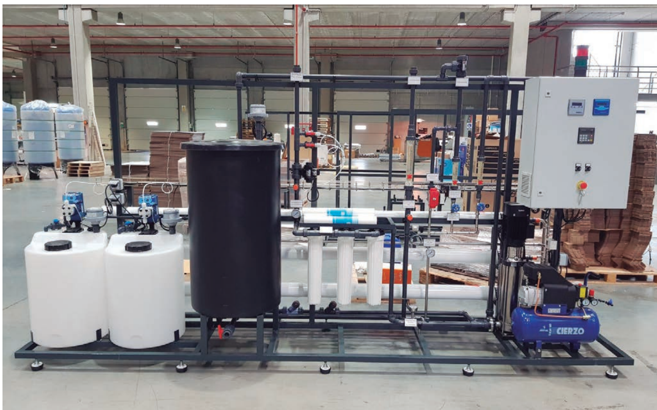
Industrial Reverse Osmosis of 43.000 l/day for the purification of drinking water in a chicken farm installed in L rida (Spain).
