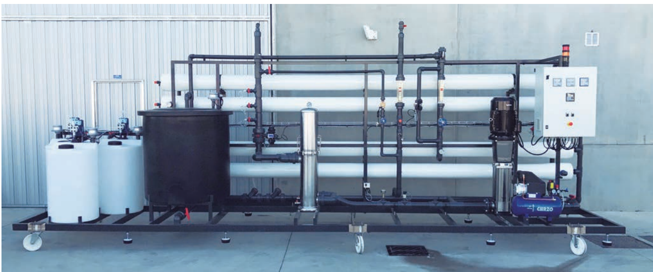
Industrial Reverse Osmosis of 400.000 l/day for a steam boiler treatment installed in Relizane (Argelia).
